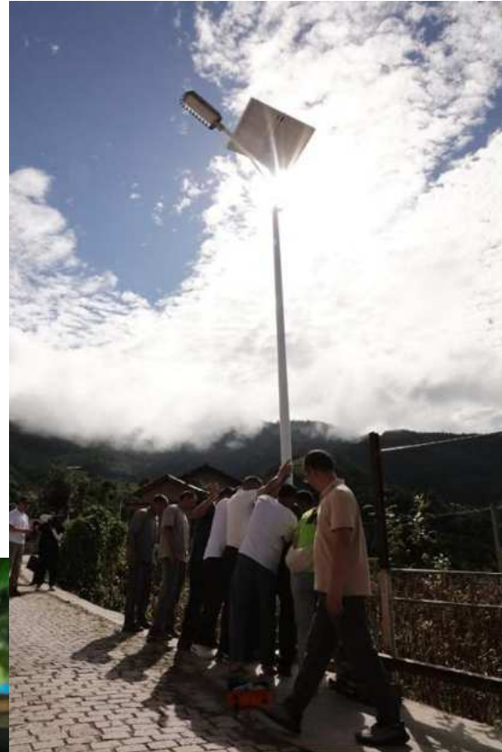
Sowers Action × EWB Hong Kong Solar Lighting Community Service Project in Yunnan
